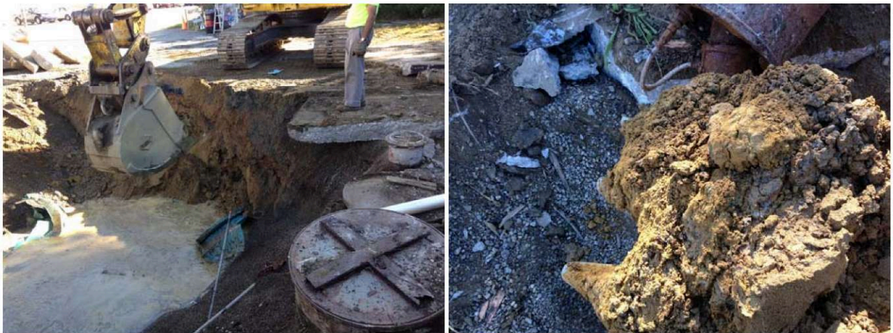
Photos 24&25 (9/24/2014): Showing collection of soil sample SW-E (left) and soil of the sidewall which exhibited no obvious staining.
