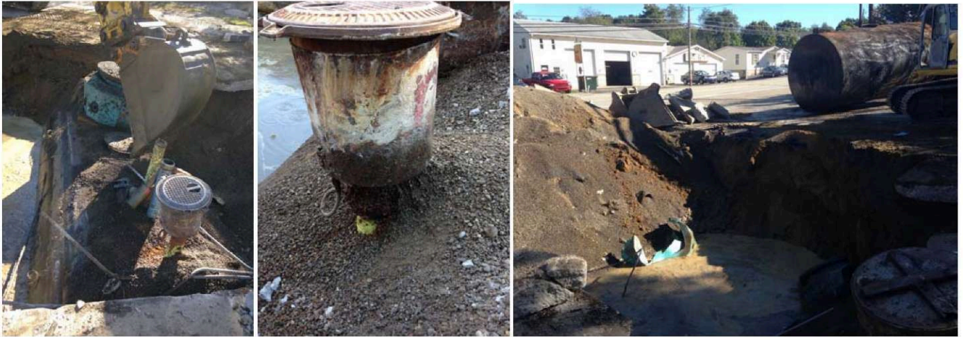
Photos 19,20&21 (9/24/2014): Tank #2 was uncovered and removed from the cavity. Significant corrosion was noted on the metal spill bucket at the fill riser with rusty staining below. The tank was found in poor condition with deep corrosive pitting, though no obvious holes were observed.
