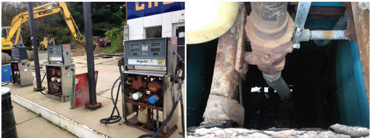
Photos 4&5 (9/22/2014): Gasoline dispensers associated with USTs #1 & 2 were fitted with under dispenser containment sumps (UDCs). All residual fluids were evacuated from the sumps using a drum-top vacuum prior to excavation activities.
