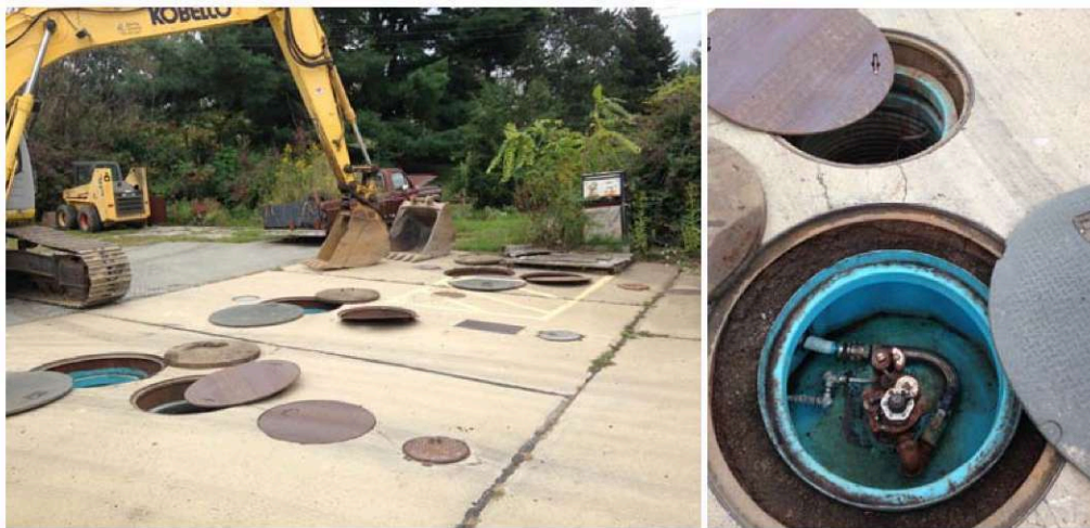
Photos 2&3 (9/22/2014): View over the tank cavity prior to excavation activities. UST systems #1, 2, and 3 utilized pressurized pumps with containment sumps at the pump heads on top of the tanks. Product lines were disconnected inside the sumps and all product was recovered from the lines using a drum-top vacuum.
