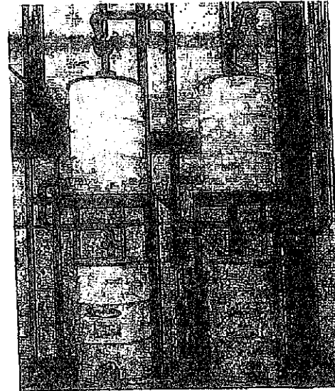
Four VentSorb units at a chemical plant are installed to operate in series end in parallel. More than 25 odorous and/or toxic vapors are controlled by 20 VentSorb units at this plant.
