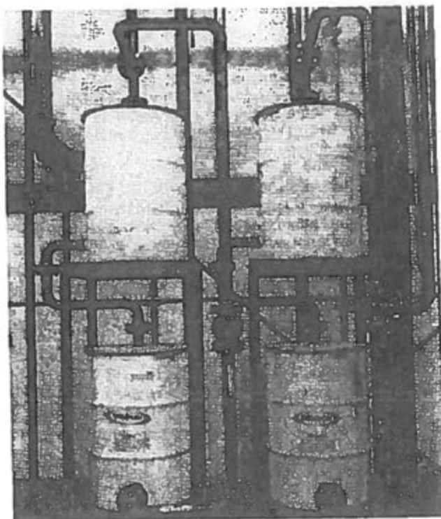
Four VentSorb units at a chemical plant are installed to operate in series and in parallel. More than 25 odorous and/or toxic vapors are controlled by 80 VentSorb units at this plant.
